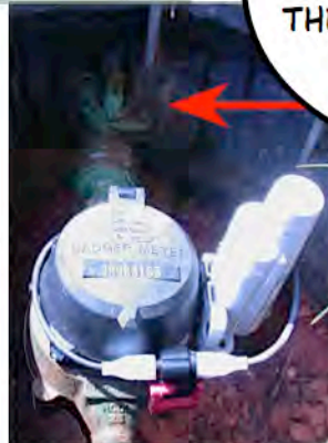
(RIGHT) MAIN SHUTOFF NEAR STREET
