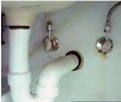
(ABOVE) SHUTOFF VALVES BENEATH SINK
